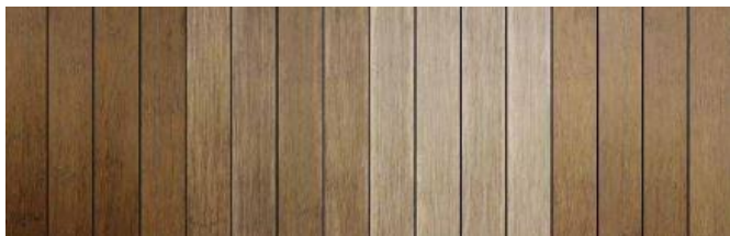
After installation After 1 year After cleaning After maintenance
